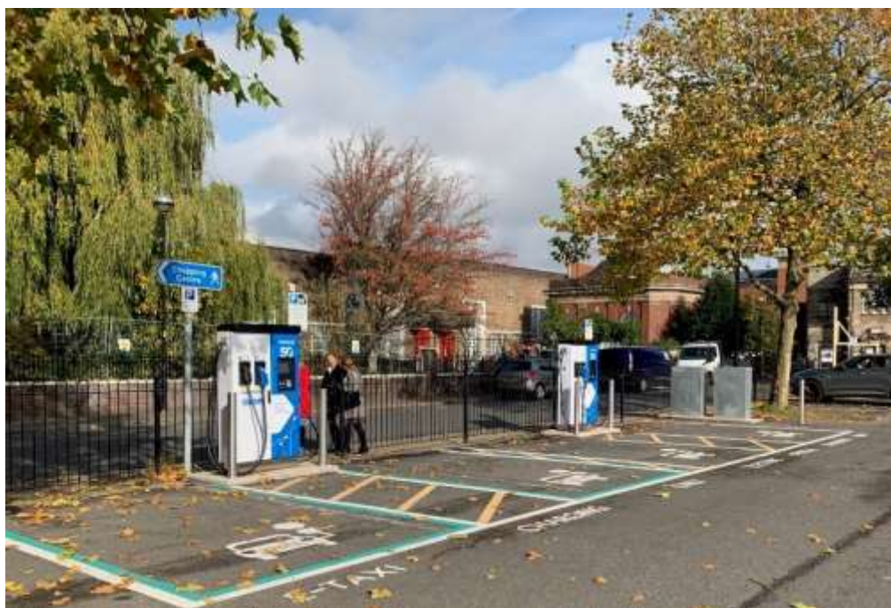
Image 17 - EV Charging Units, King Street Car Park Stoke-upon-Trent
