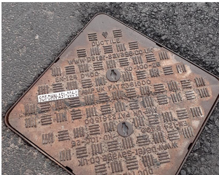
Figure 10 - Example of identifying tag attached on the chamber lids.
